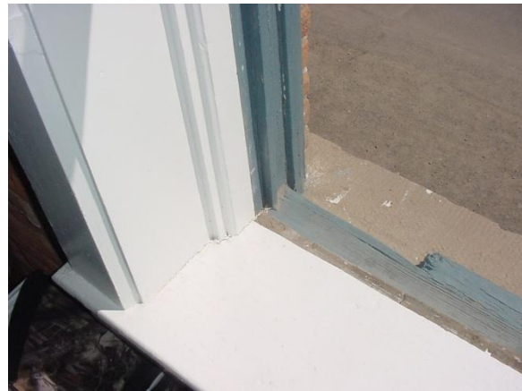
Upper level window: damaged wood trim.
