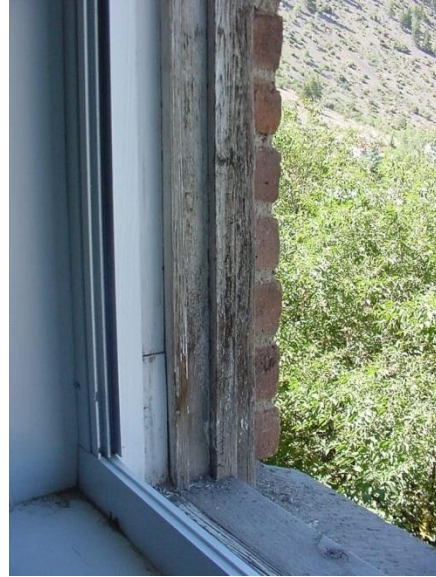
Upper level window: rotted trim.
