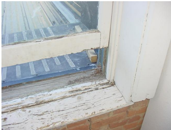
Upper level window: rotted sill
