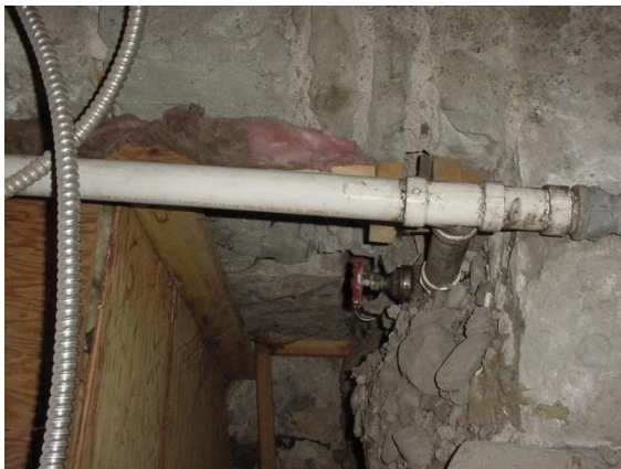
Above: Domestic water service entry. Right: Lower level pump station.
