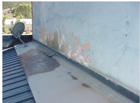
Sheet metal flashing.
