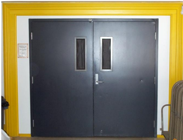
Above: Non-original hollow metal doors between theatre and lobby. Trim is original.
