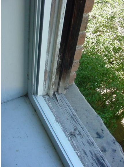
Upper level window: rotted sill.
