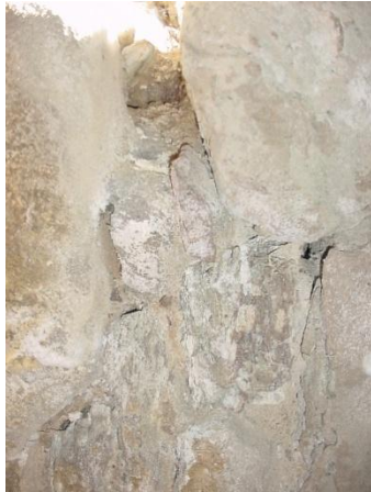
Left: Eroded area at south stone foundation wall.
