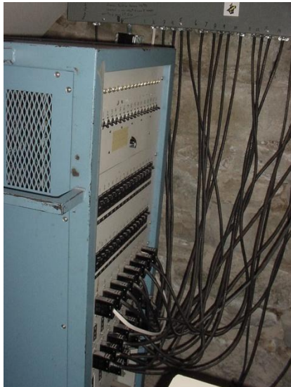
Left: Theatre load center, currently in men's dressing room.
