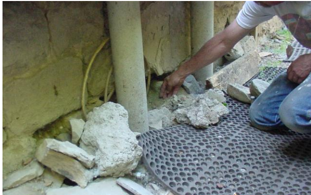
Left: Crumbling stone masonry at base of northwest corner of building 2.
