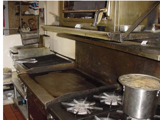
Kitchen, stove and fry top.
