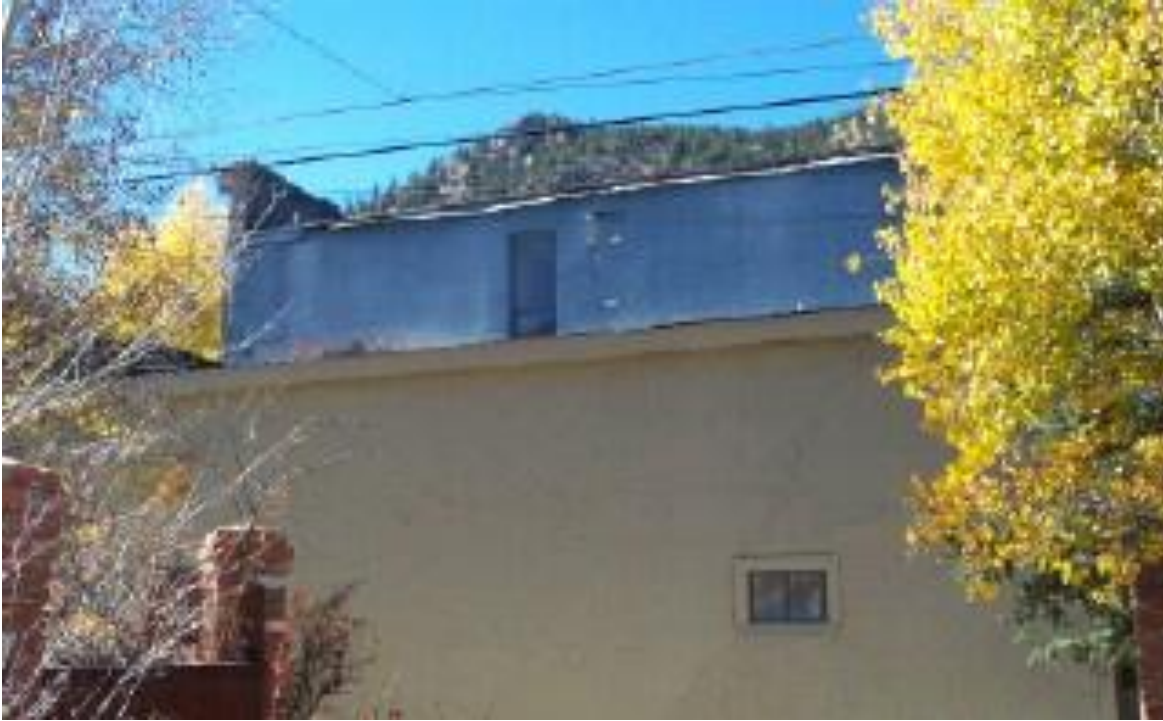
Hough Building upper portion Building 1 east elevation (partially obscured by adjoining structure).
